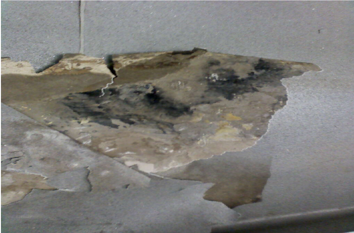
Example of mold under kitchen flooring July 2012.
