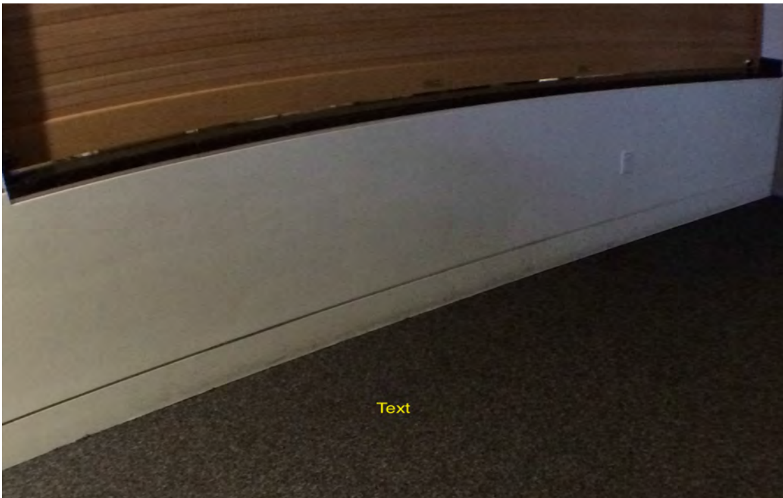
Tree room damaged walls
